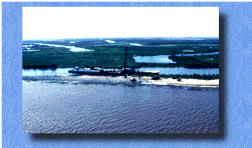
Photo 15. Project managers stabilized this narrow beach with boulders to prevent erosion of the wetlands behind it.
